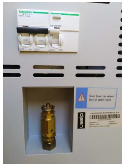
Exhaust purge valve (below).
