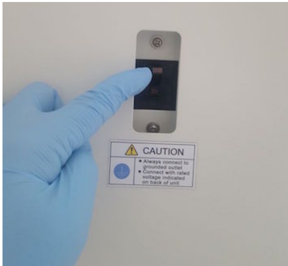
Thermomagnetic electrical switch.
