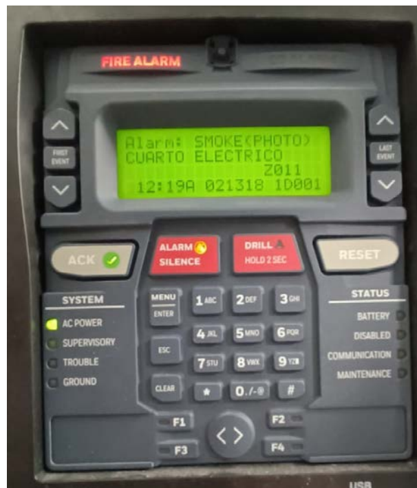
In this example, the central smart control panel indicates that the alarm was caused by smoke detection in the electrical room.
