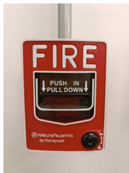
Manual activation control
