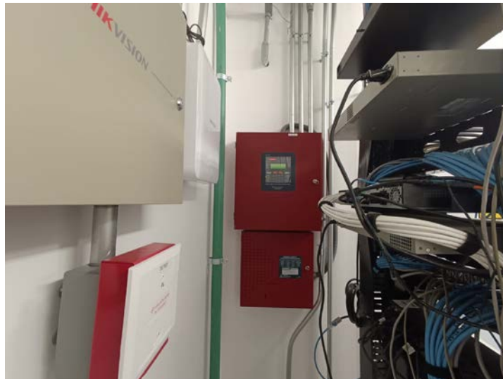
Location of the alarm's central intelligent control panel.
