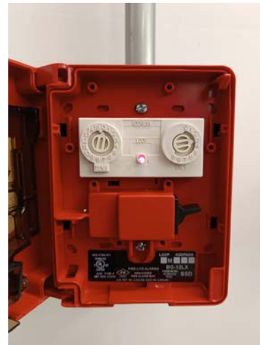
Interior del control manual.
